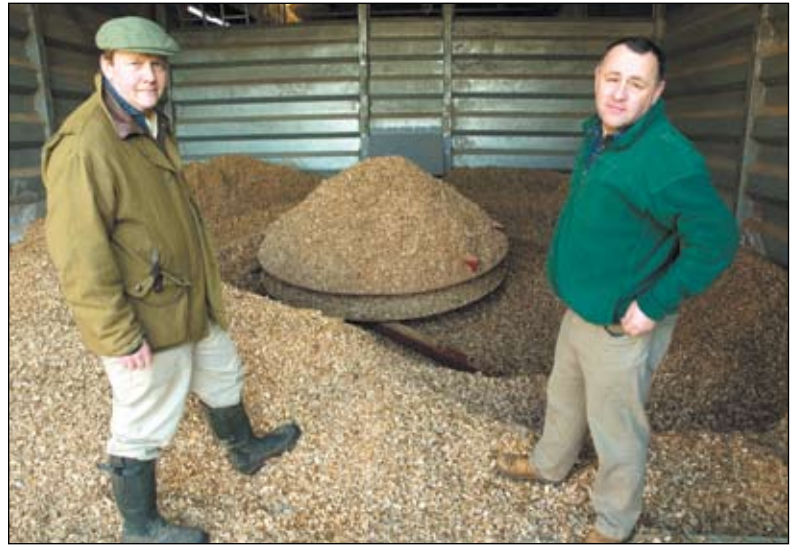
Nick Deterding and Gary Battell in the receiving pit, a converted dryer barn. The central 6.4-metre sweep collector 'sweeps' clifs of woodchip into a central auger which feeds (rotates) the chip through the back wall straight into the 550kW Gilles boiler. The barn is filled once a month during the winter.
