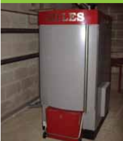
The system centres on a Gilles HPK-RA 70 woodchip boiler
