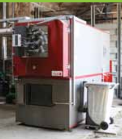
The system centres on a Gilles HPK-UTSK 550 woodchip boiler
